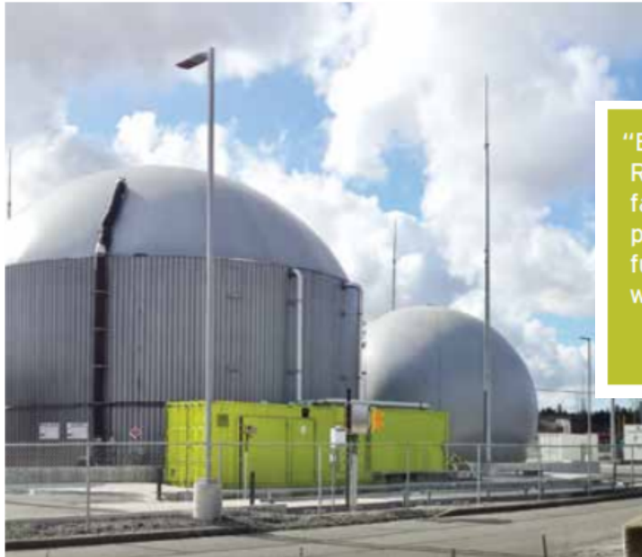
Surrey Biofuel Facility storage tanks, fermenter, and biogas buffer.
